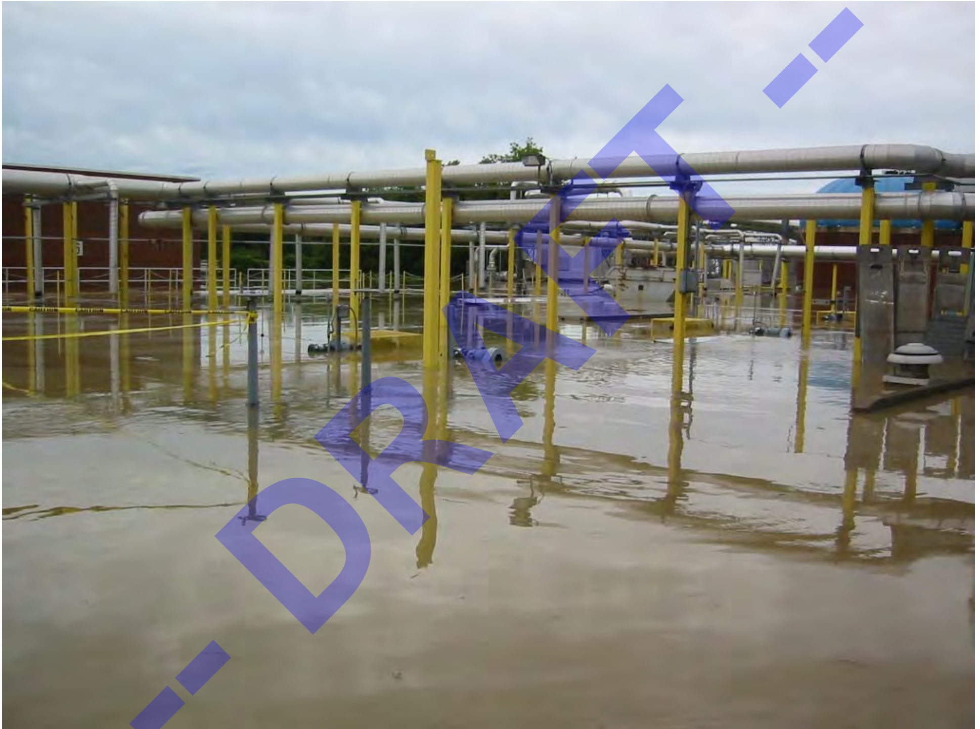
09/08/2011 @ 8:56am - internal view of flooded Joint Sewage Treatment Plant over Primary Settling Tanks (JSTP employee photograph)
