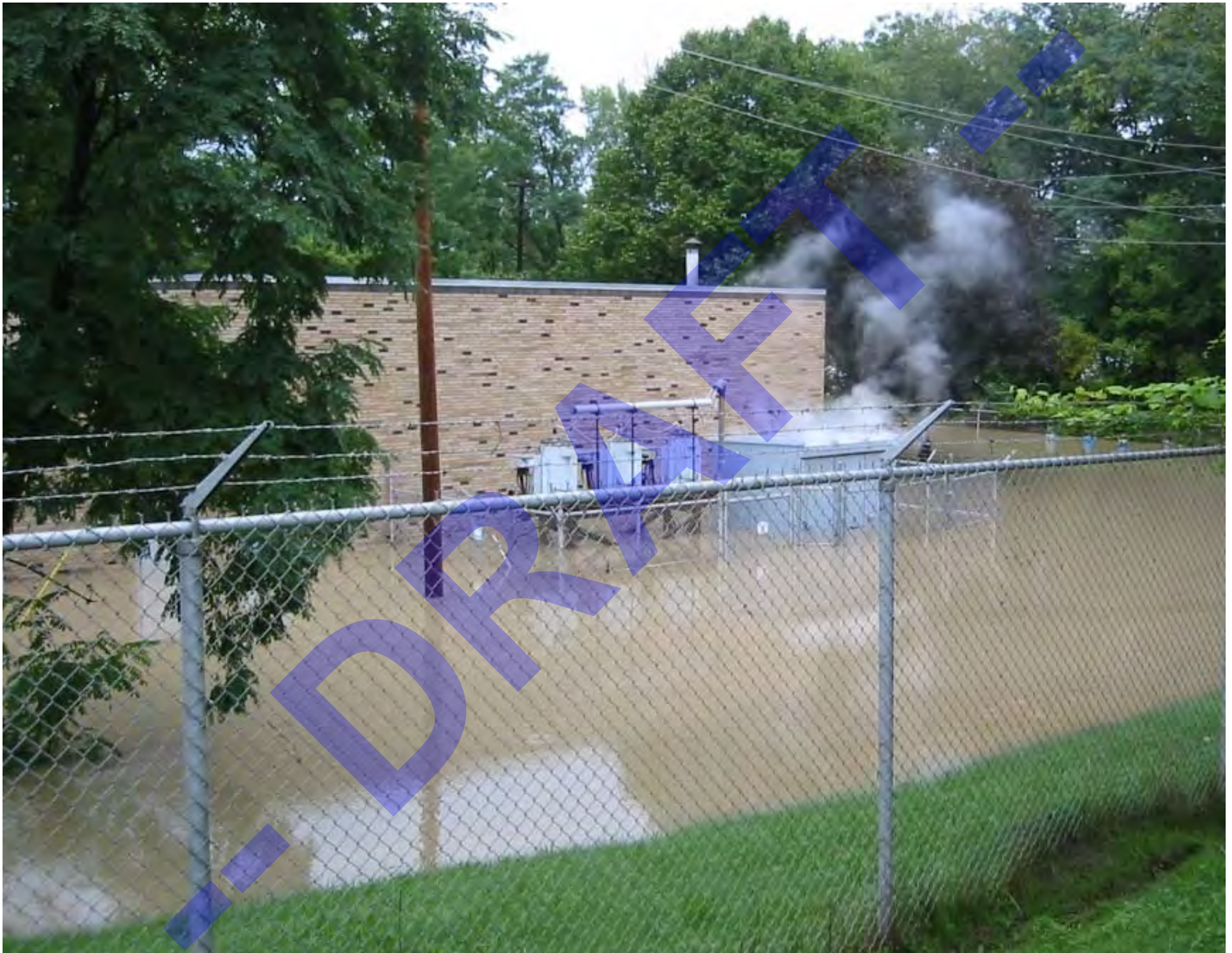
09/08/2011 @ 8:16am - view of flooded Terminal Pumping Station with external electrical components steaming from exposure to flood waters (JSTP employee photograph)
