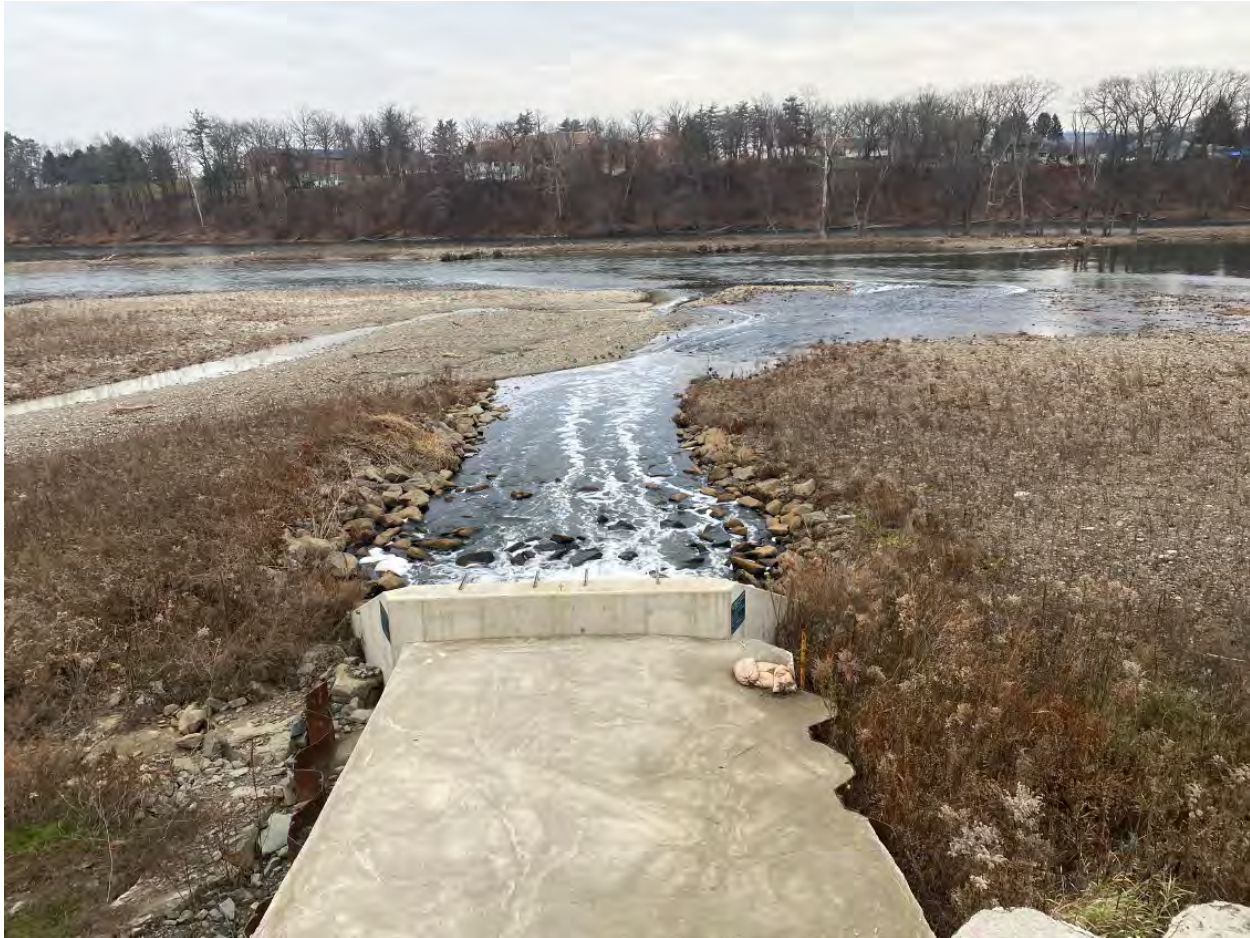
Figure 2: Outfall 001 at BJCSTP.
