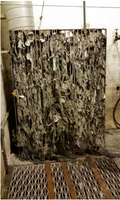
One of the Gratings covering the channel grinders.
