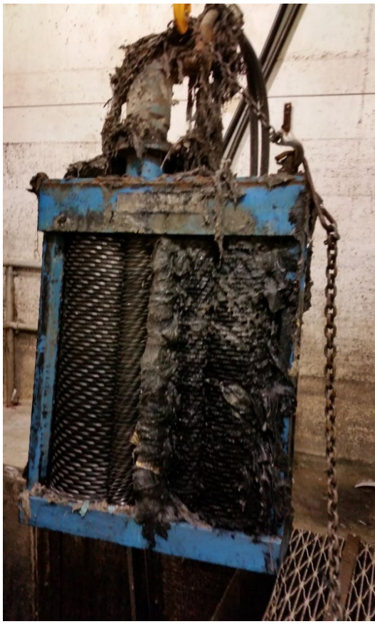
One of the TPS Channel Grinders being removed to unclog.
