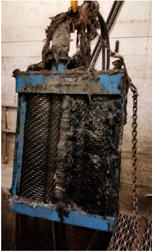
One of the TPS Channel Grinders is being removed to unclog.
