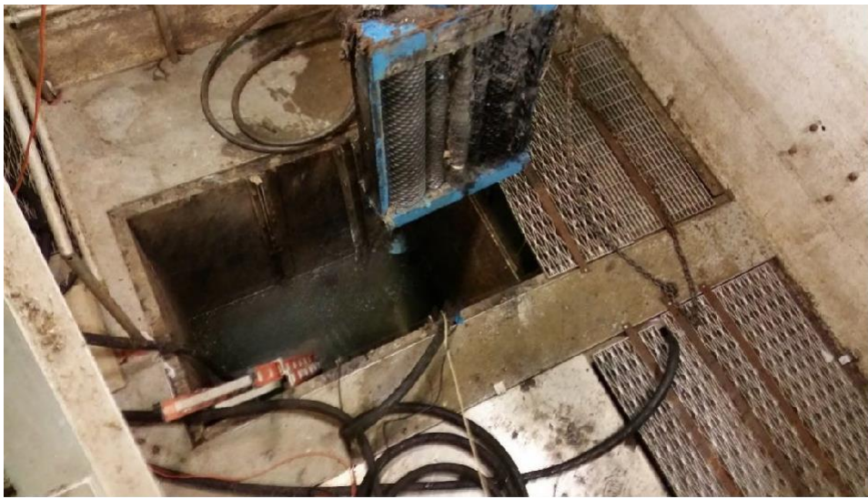
Channel Grinder being removed from West Channel at Terminal Pump Station (TPS)
